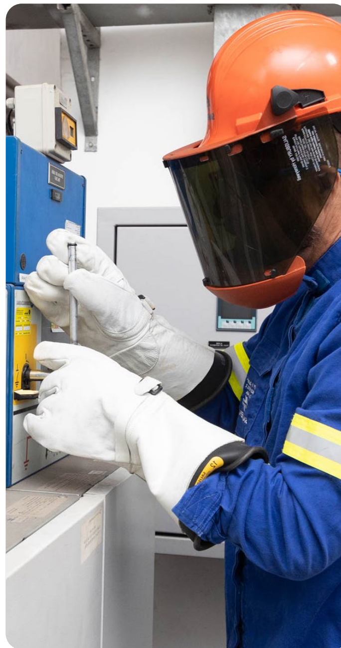
Corte Branco Reservoir electrical system - Photographer: André Thiago Chaves Aguiar
